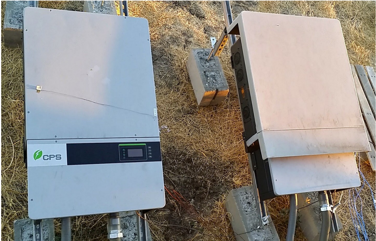
Figure 2 Image of the installations of the two (2) CPS SCA28KTL-DO/US-480 – the inverter on the right-hand side of the image has a shade cover installed
