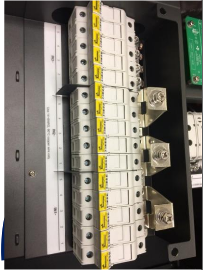
Figure 9-4 Bypass Terminals Installed on NEG Bus
