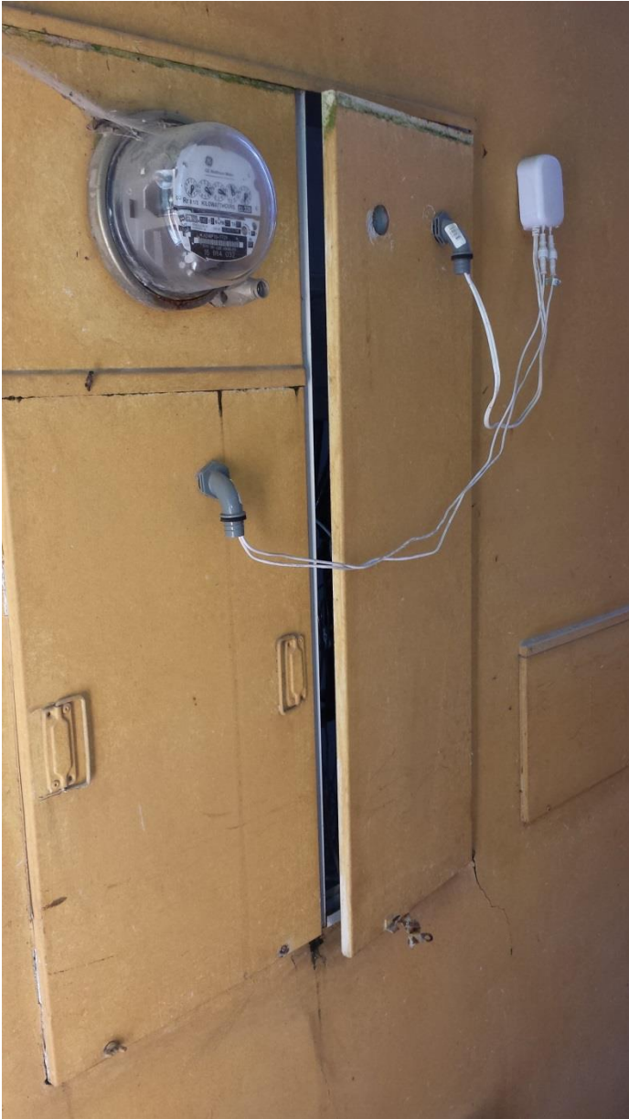
Figure 1 Gen5 HEM Installation
