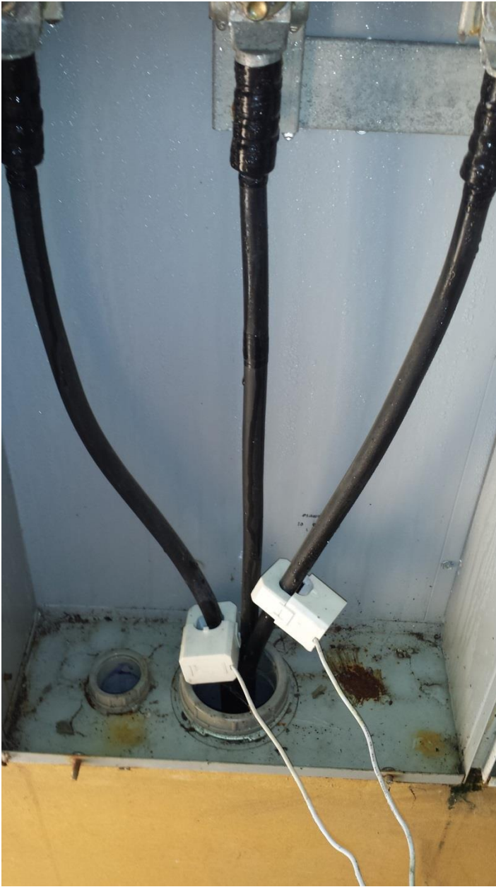
Figure 2 Example of a valid CT Clamp Position
