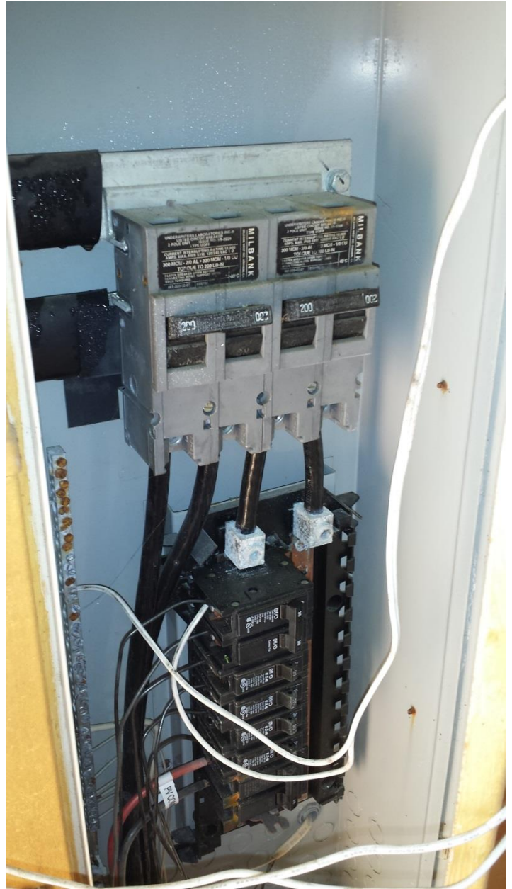
Figure 3 Example of 120V Voltage Sense Connection
