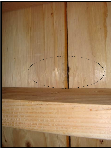
Figure 4a. Buckled Plywood Shear Perpendicular to Rafter
