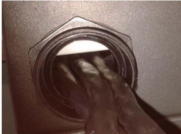
Figure 4.2 – AC Side Knockout Partially Blocked
