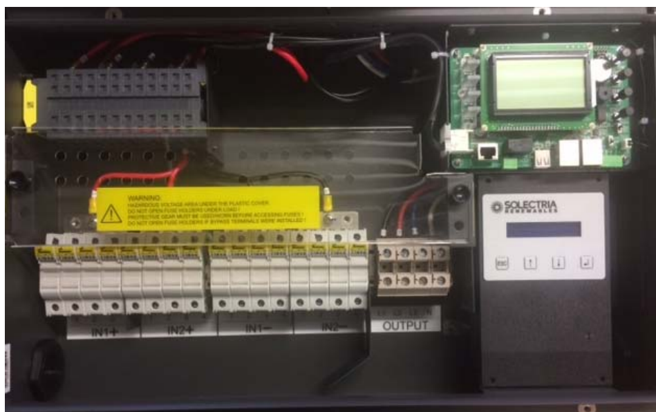
Figure 14.3 – SolrenView Monitoring Installed Inside Wiring Box
